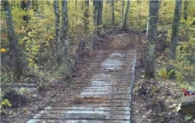
Concrete boat planks used in Nemadji State Forest to harden a wet trail crossing.
