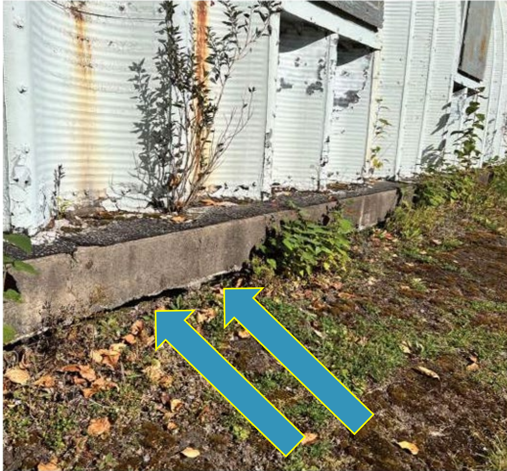
Erosion along thickened edge slab foundation has exposed the underside of the structure.
