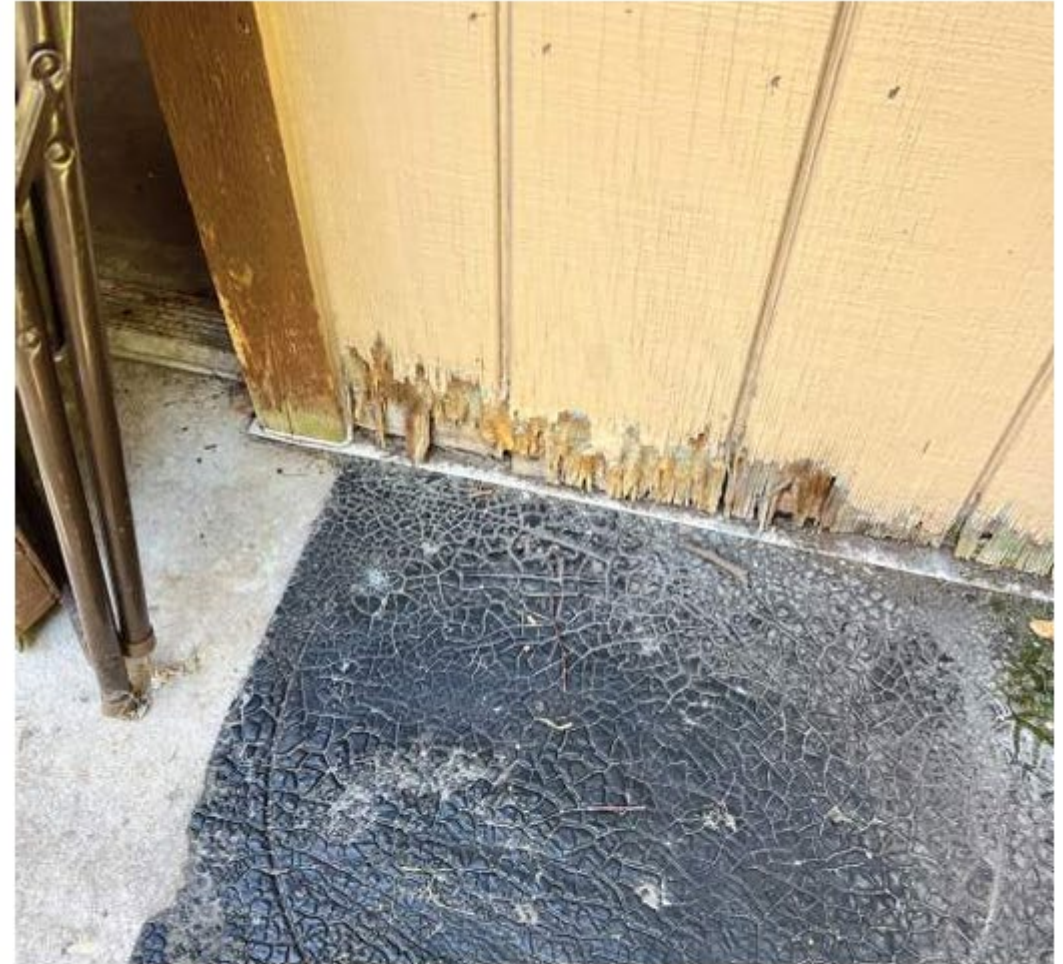
Deteriorated T1-11 siding has notable moisture intrusion.
