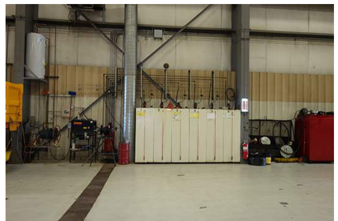
Below: A view of the lube storage equipment and pressure washer area.
