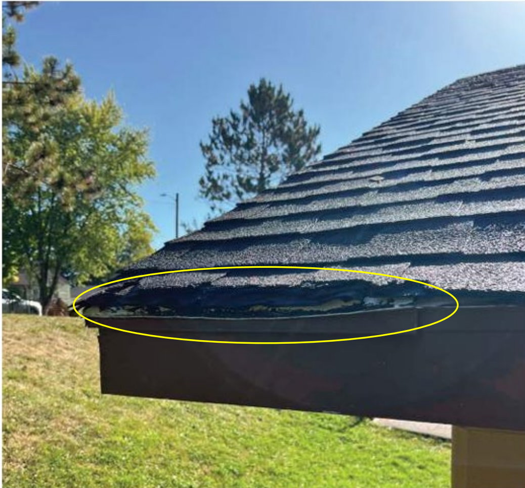
Asphalt shingles missing and delaminated - in need of replacement. Condition of substructure not assessed.
