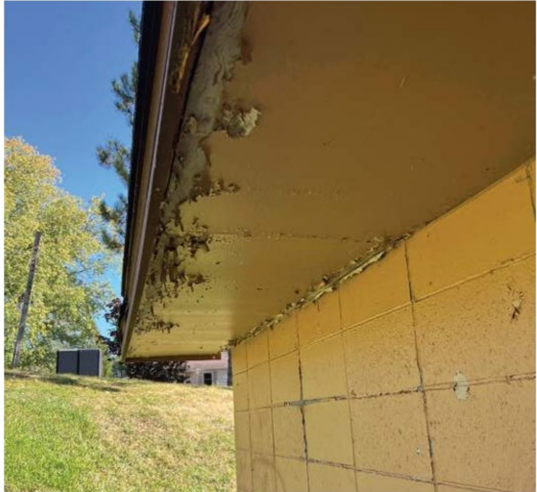
Painted wood soffits and fascia are beyond their useful life and in need of replacement.
