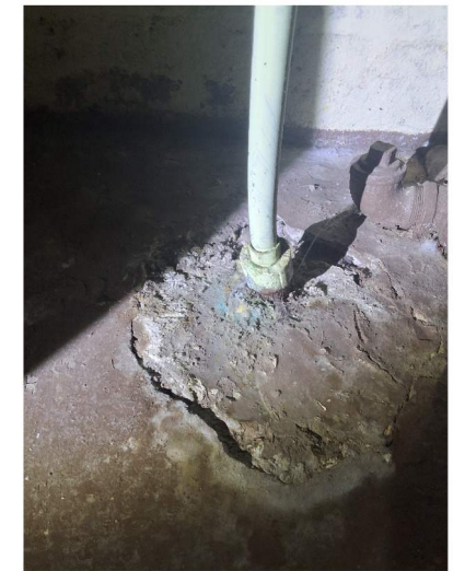
WATER SERVICE PIPE
