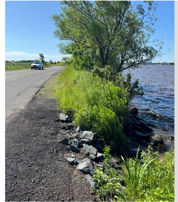
Figure 02.35 Existing narrow shoreline with erosion
