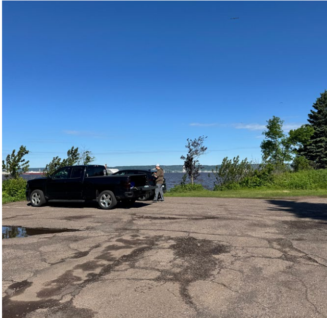
Figure 02.18 Trailer parking flooding (left)
