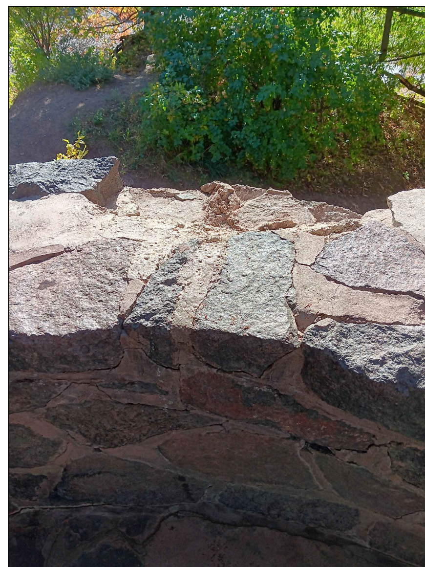
EAST TOWER DETERIORATED WINDOW SILL
