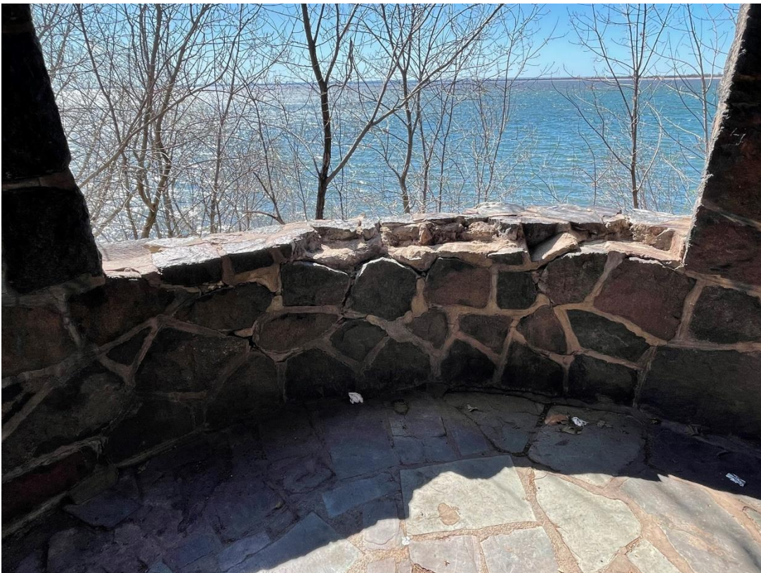
Photo 10: View of missing stones on the sill of West tower wall opening.
