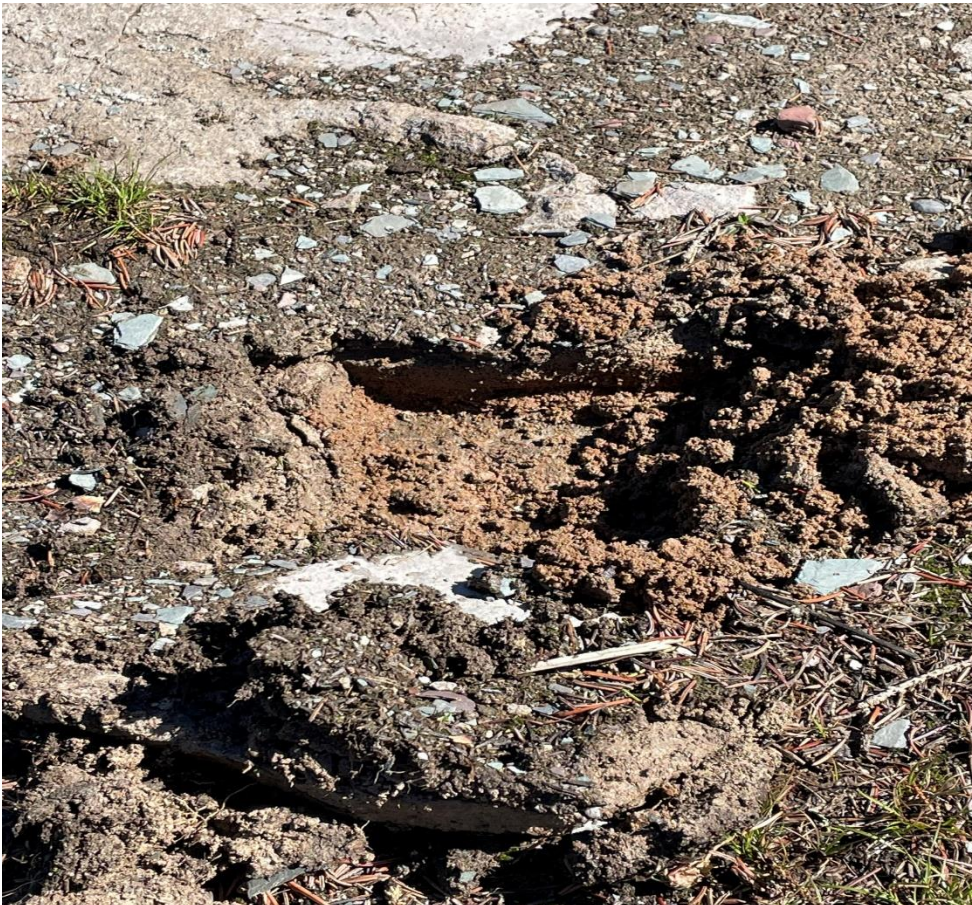
Photo 12: Example of dirt and debris (mud) building up on top of the concrete structural slab due to missing field stone.
