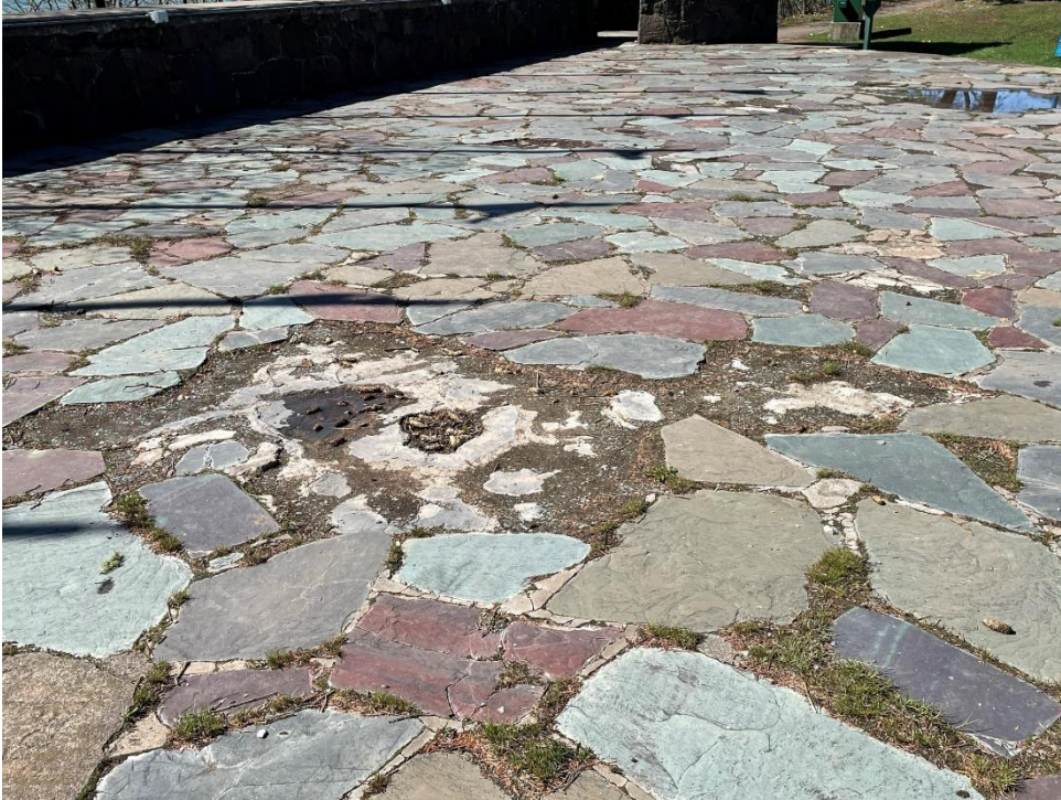
Photo 11: View of missing field stones and ponding water on the stage surface.
