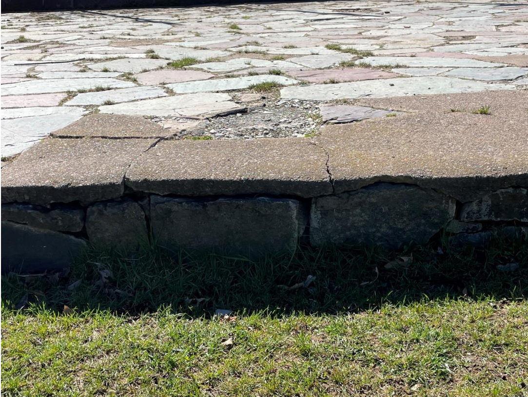
Photo 9: Example of the displaced/loose stones evident on the stage north stone wall.
