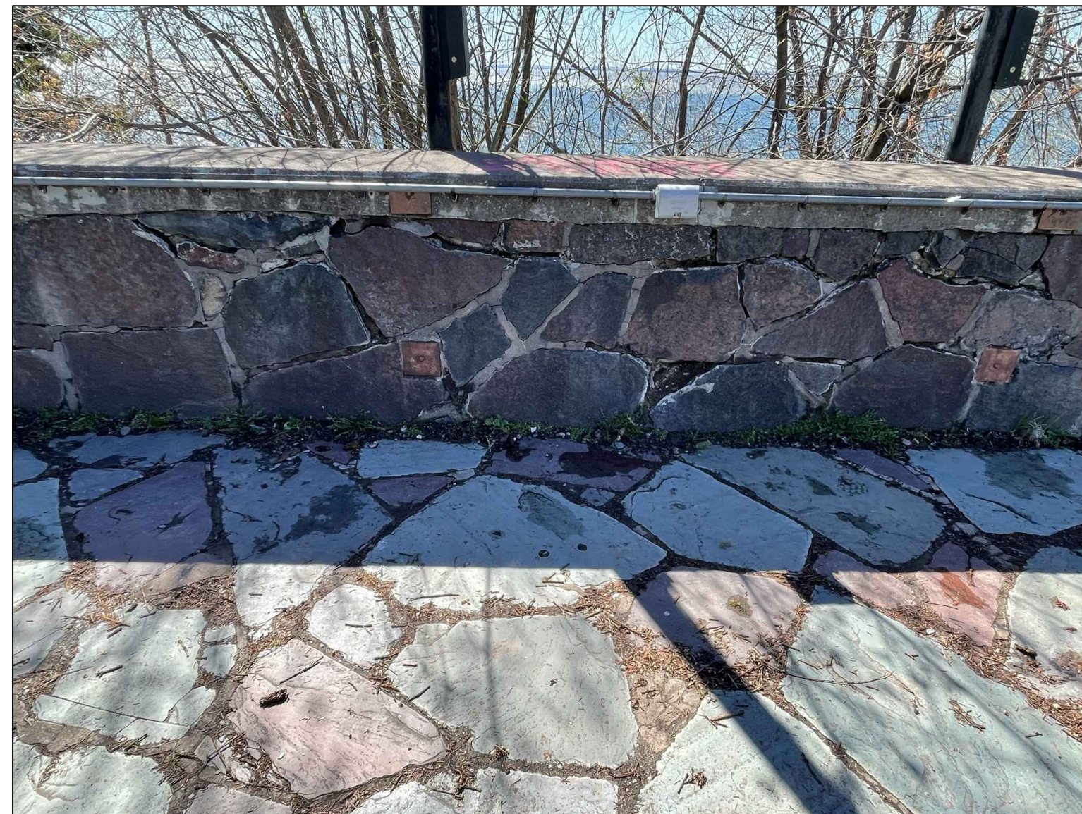
FRONT VIEW OF BACK STAGE WALL DETERIORATED MORTAR JOINTS
