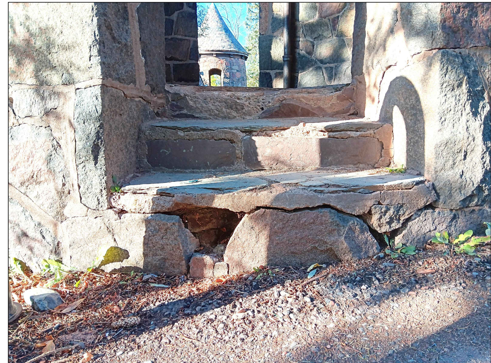
EXISTING EAST TOWER DETERIORATED ENTRY STEP
