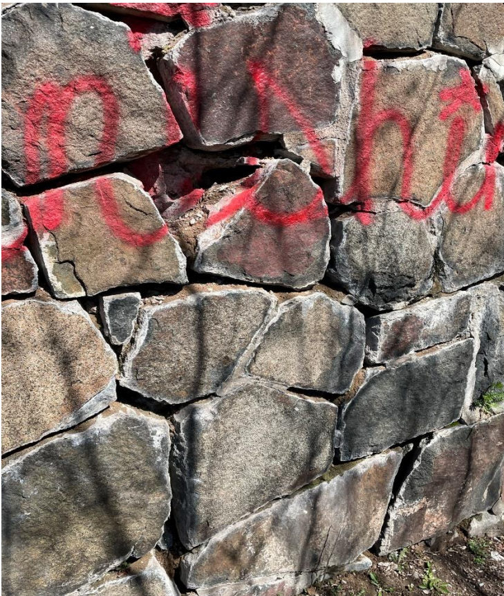
Photo 8: Example of missing stones/void spaces present in the stone walls, photo on south wall face.
