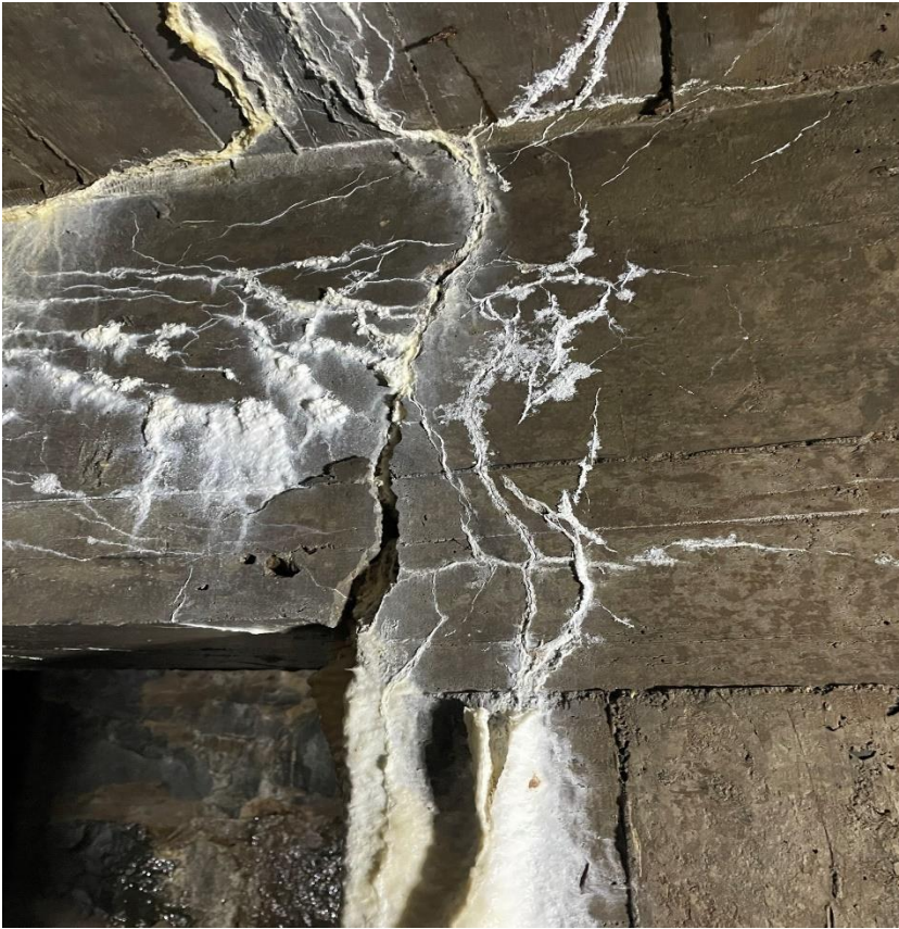
Photo 5: Vertical crack in concrete beam below the stage.
