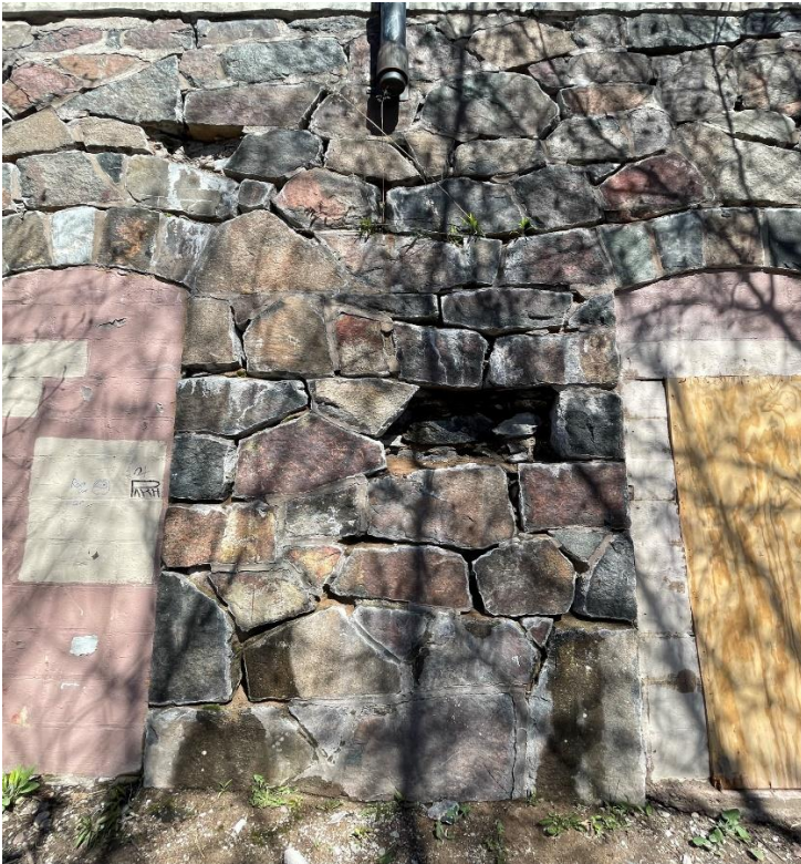
Photo 7: Exterior face of south stone wall. Note missing stones and decayed mortar joints present.
