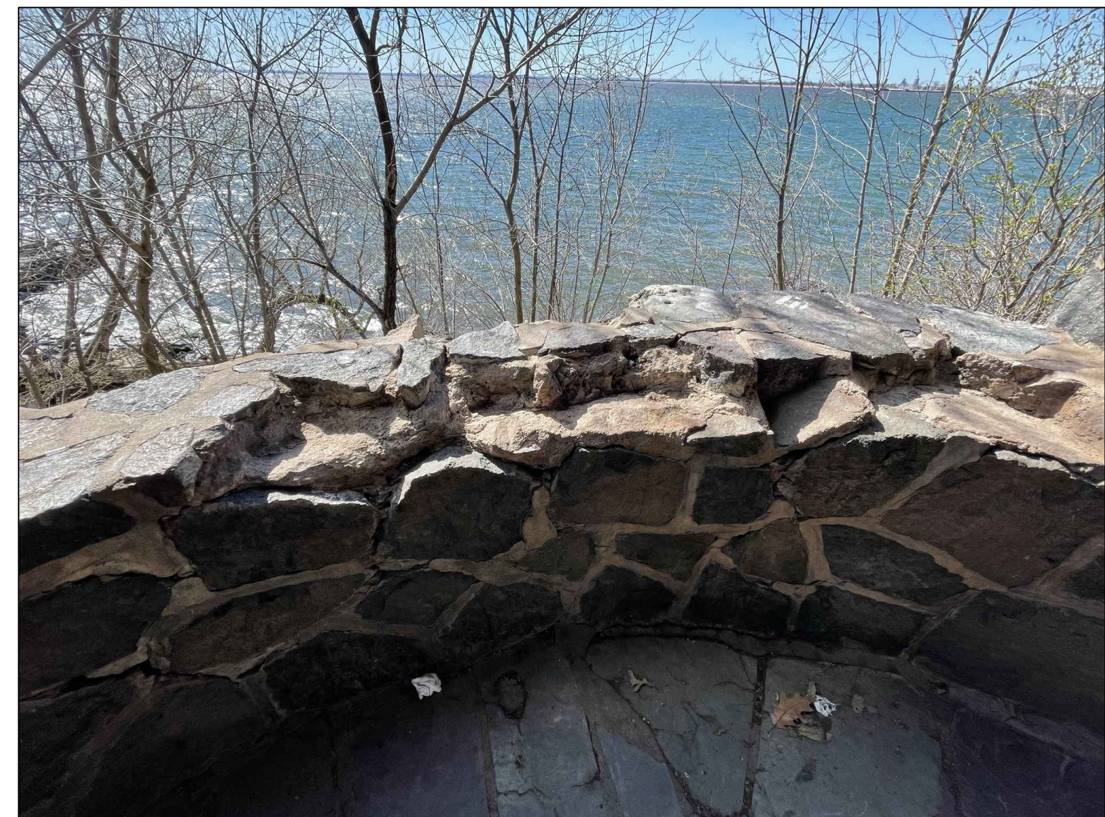
WEST TOWER DETERIORATED WINDOW SILL
