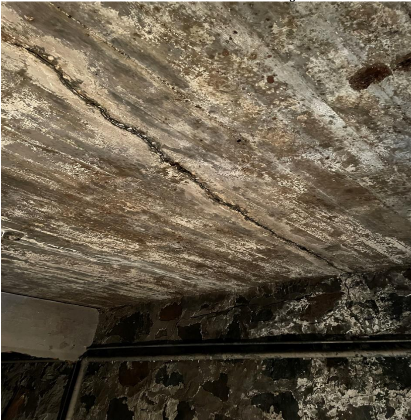
Photo 6: Crack in stage slab from below. This does allow water to leak into the basement area.
