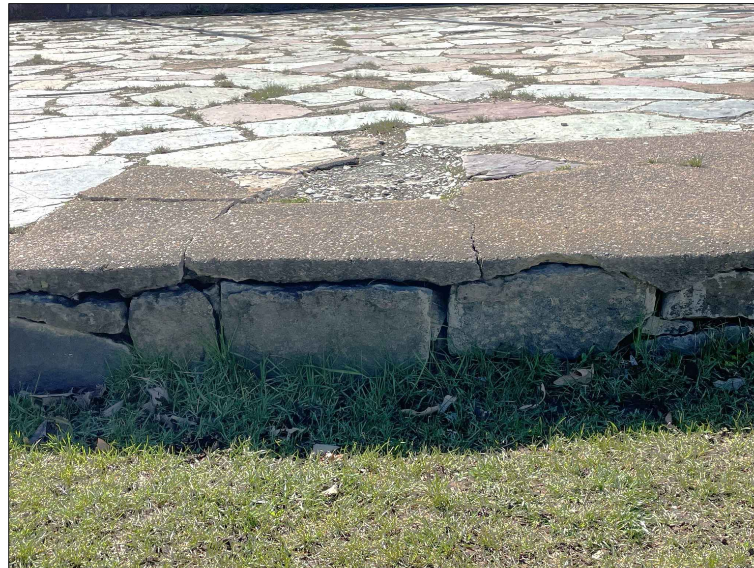
TYPICAL STAGE FRONT WALL DETERIORATED MORTAR JOINTS
