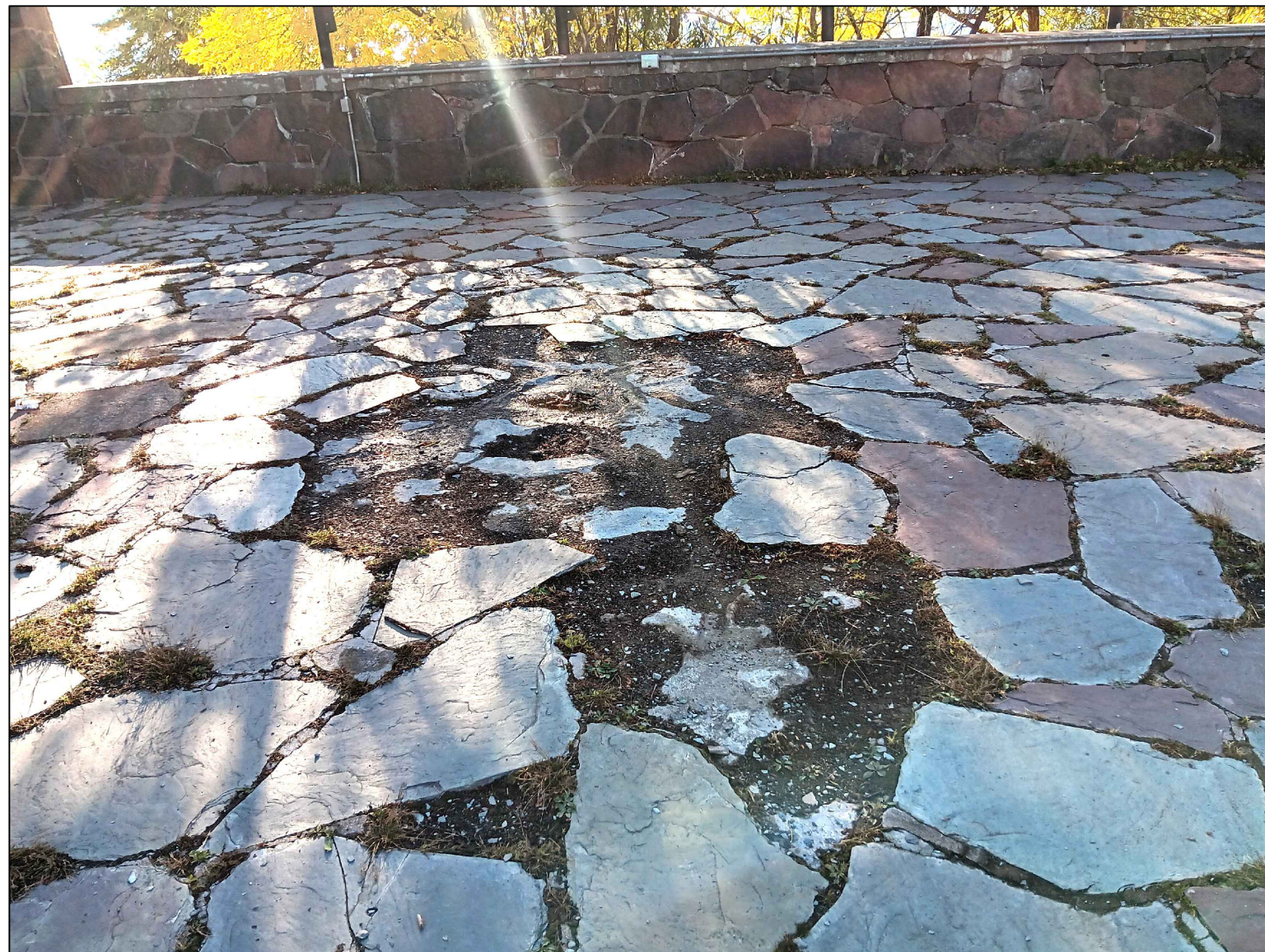
TYPICAL PHOTO OF DETERIORATED STAGE FIELD STONE
