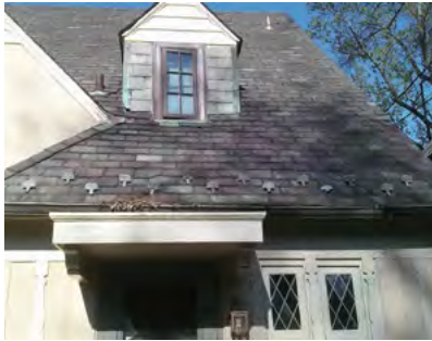
[8] Regular maintenance includes removing leaves that can clog gutters and cause water damage to the exterior and interior walls of a house.
