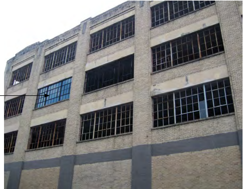
[19] Installing a mockup of a proposed replacement window can be helpful to evaluate how well the new windows will match the historic windows that are missing or too deteriorated to repair.
