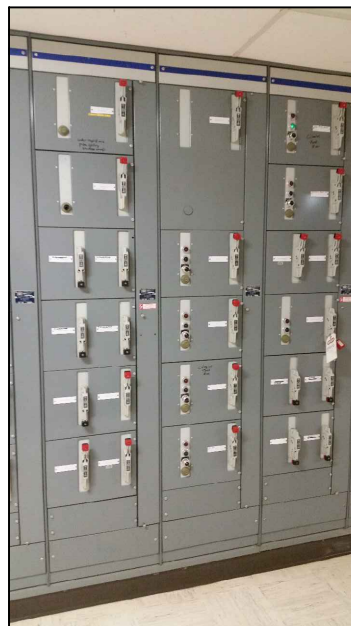
6 EXISTING WTP-MCC-A TO REMAIN
