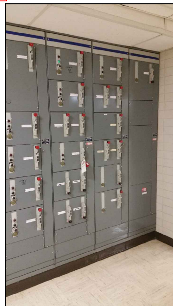
7 EXISTING WTP-MCC-A TO REMAIN
