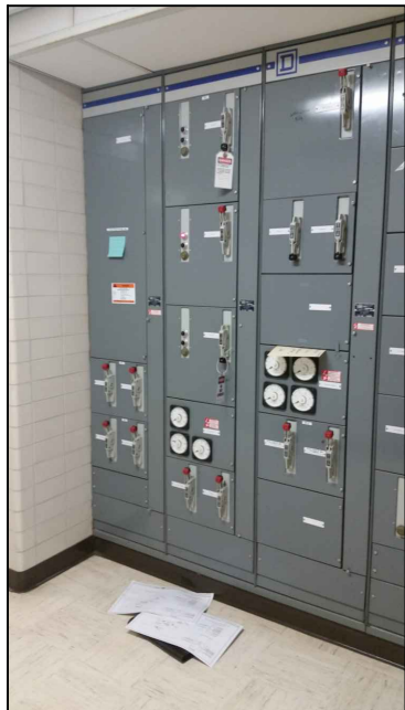
5 EXISTING WTP-MCC-A TO REMAIN
