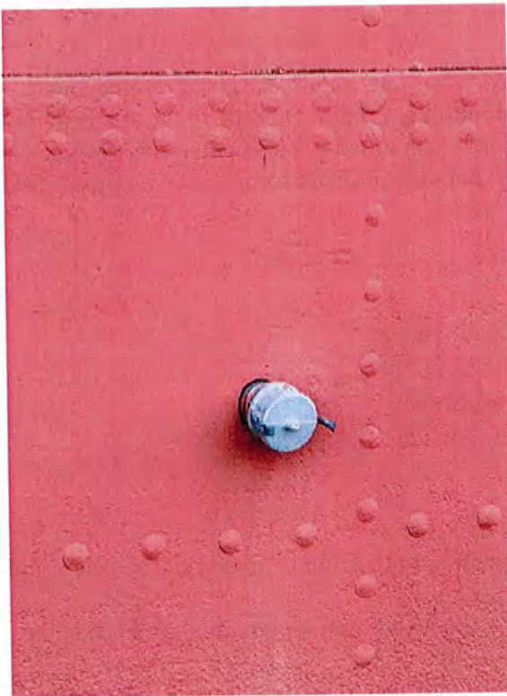
Number 5 Port – Sewage overboard
