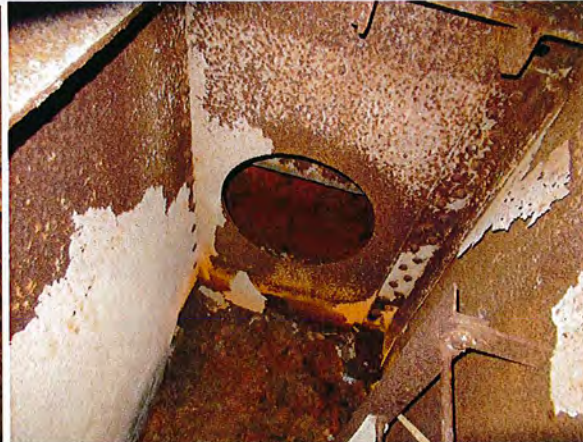
Lightning hole and water accumulation
