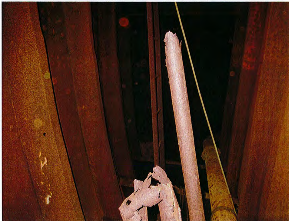
Completely deteriorated sounding pipes
