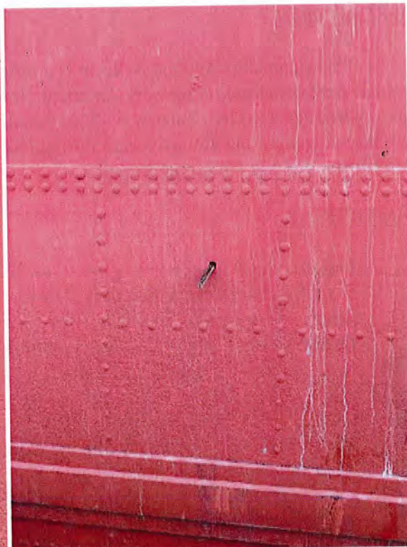
Number 6 Port – Through hull penetration
