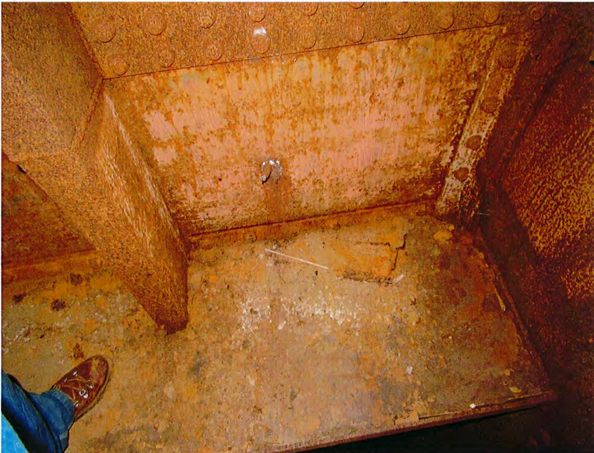
Hole burned in side shell
