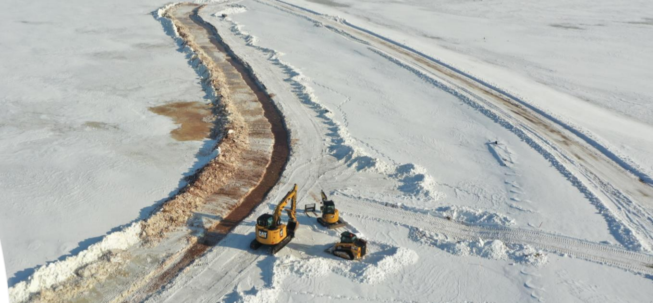
January 2023: A trench is made adjacent to the Delta Upland Cap to place logs for shoreline protection.
