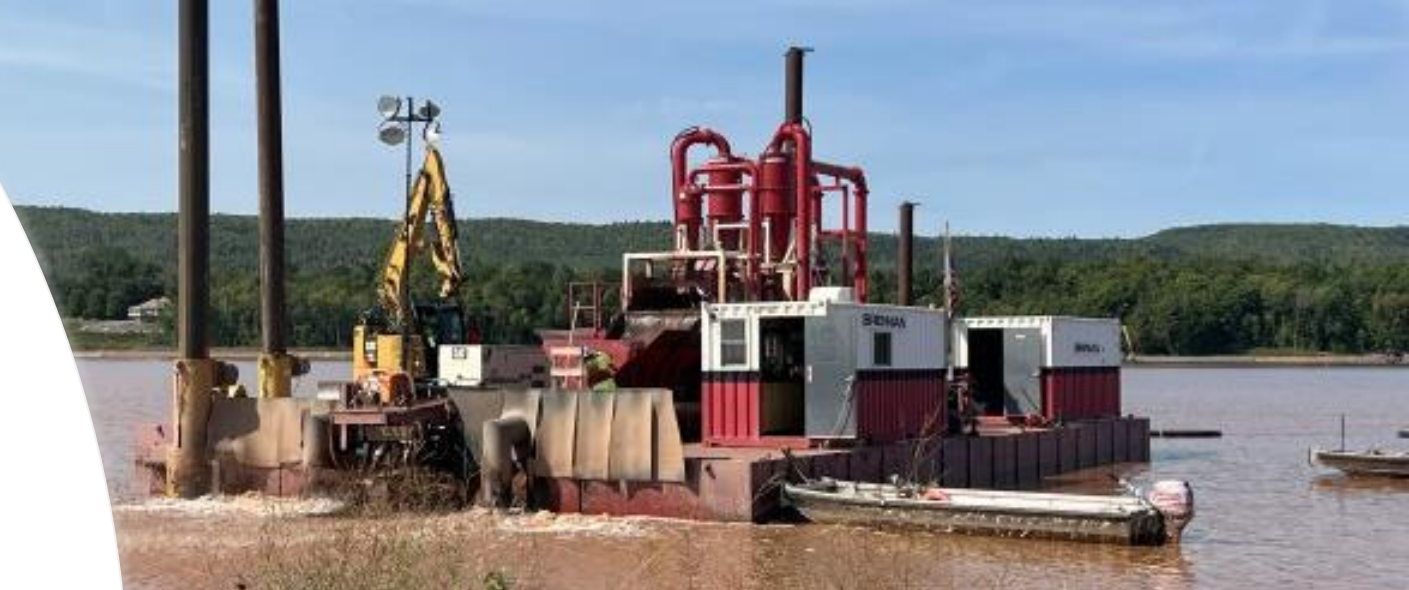
September 2022: A capping barge places material in the Shallow Sheltered Bay near the spit of land.
