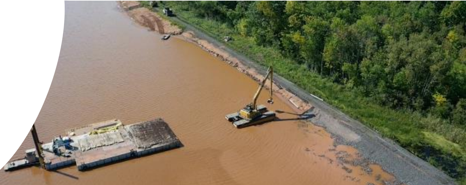
September 2022: Erosion control straw matting is placed on the shoreline of the Shallow Sheltered Bay to protect the soil and seeded areas.
