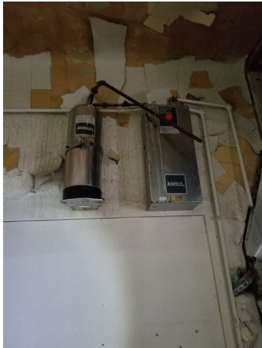
Chemical Fire Suppression System
