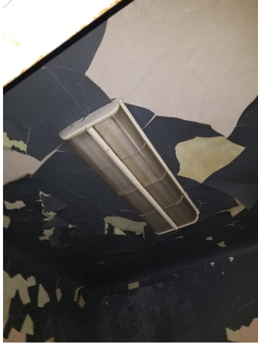
PCB Containing Lights
