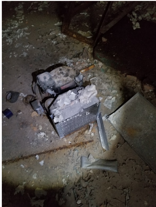
Discarded Refrigerant Pump
