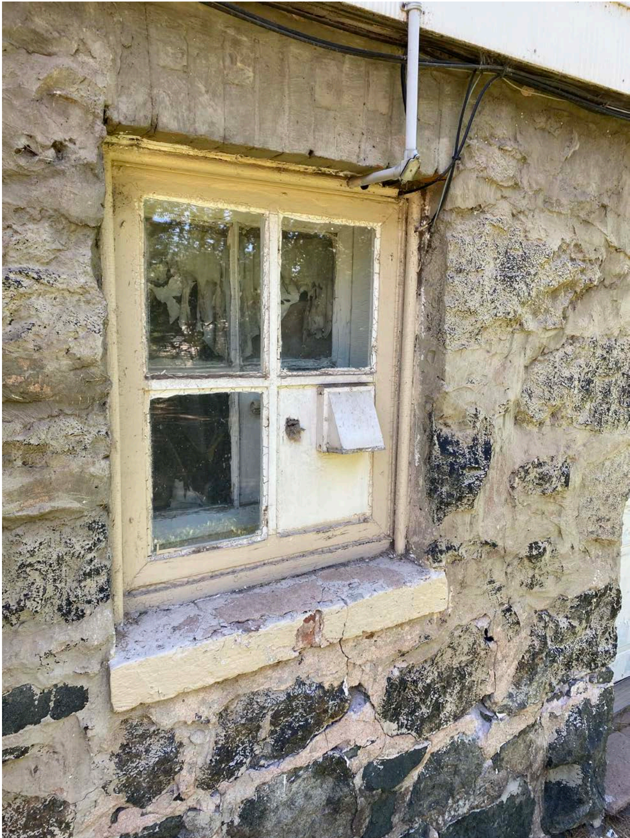
Photo 0011: View of wood window and stone foundation at west elevation, looking southeast.
