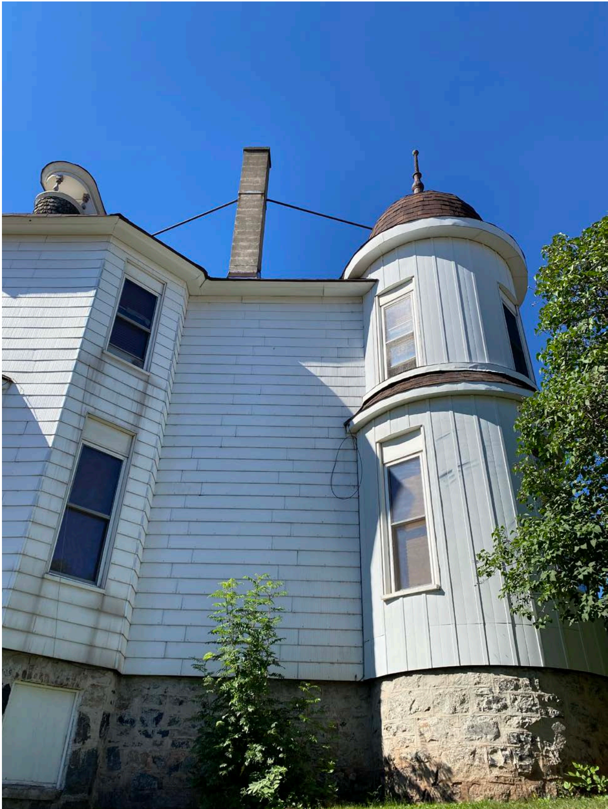
Photo 0015: View of tower, chimney, and dormer at the east elevation, looking west.
