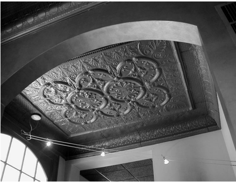
Decorative pressed metal ceilings like this example at the Gardner House are found on the interior of many commercial buildings in Hastings.
