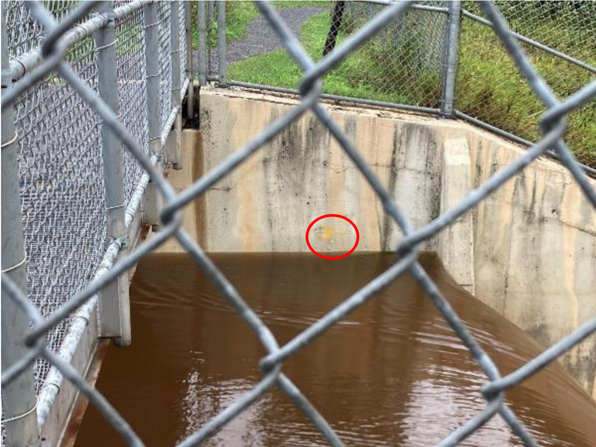
Figure 12. Stage over Hartley Dam Spillway (note stage marking over the spillway- circled in red).
