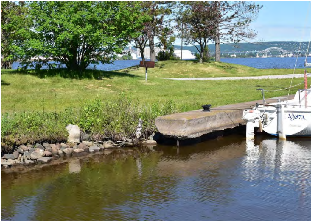
Photo 2: Park Point Harbor showing undercutting of bulkhead and shoreline erosion.
