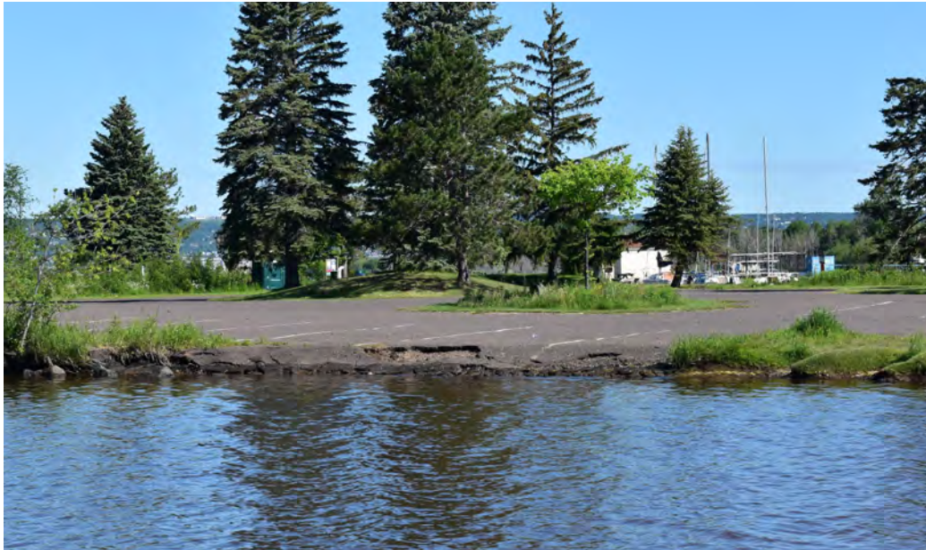
Photo 1: Park Point Harbor showing subsidence of parking lot.
