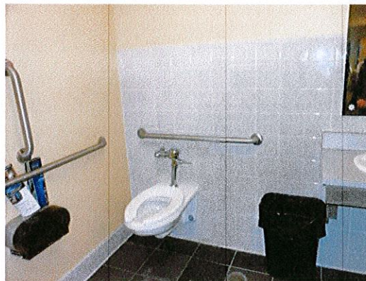
Photo 5: The attached police station provides accessible toilet and shower facilities.
