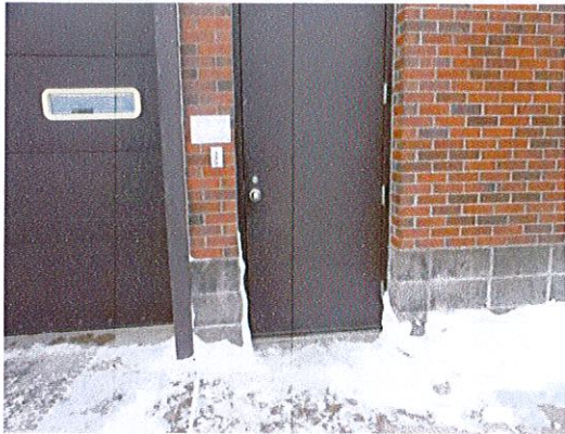
Photo 1: Service door to apparatus area. Replace the knob with a style that does not require grasping, pinching or twisting to operate (such as a lever).
