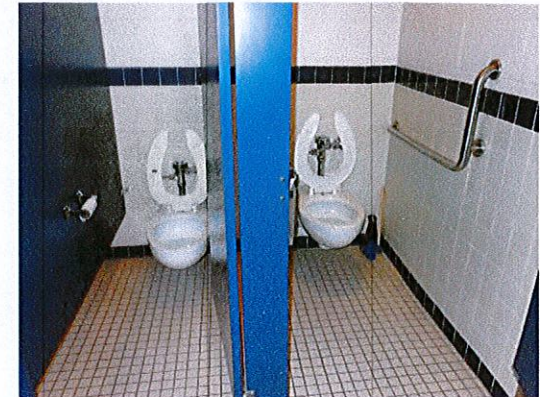
Photo 3: View of toilet room. An ambulatory accessible stall is provided, but not a stall with 60" clearance.
