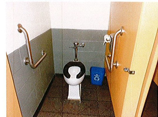
Photo 6: The toilet rooms provide an ambulatory accessible stall, but not a 5' accessible stall.
