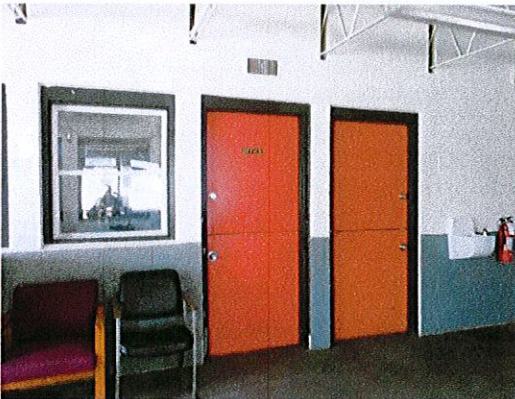
Photo 4: Typical door hardware throughout the building is a knob style. Replace the knobs with a style that does not require grasping, pinching or twisting to operate.
