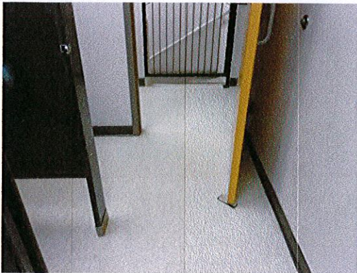
Photo 4: The stall partition currently obstructs the maneuvering clearance at the entry door to the women's toilet room.
