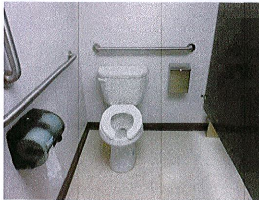
Photo 5: The toilet room has been remodeled to increase accessibility. Relocate the sanitary waste receptacle to below the horizontal grab bar. Note: the stall is only 51" wide (vs. 60" due to fixture count).
