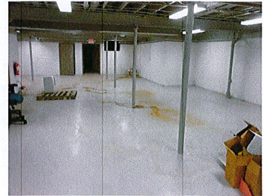
Photo 6: View of lower level. The lower level is currently abandoned and used only for storage. There is not an accessible route to the lower level.
