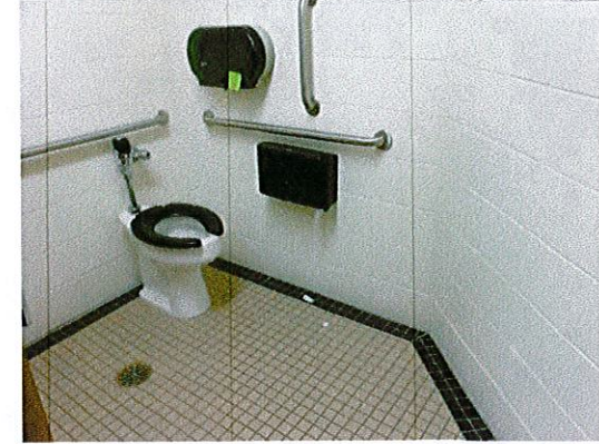
Photo 9: View of upper level women's toilet room. Remove the 2nd toilet paper dispenser currently mounted above the grab bar. This location does not currently provide 48" in front of the toilet due to the angle of the exterior wall.
