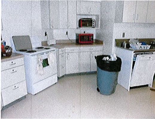
Photo 7: View of kitchen. Currently no features of accessibility have been provided.
