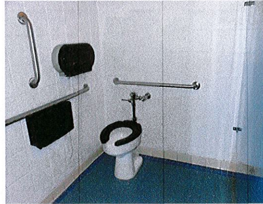
Photo 8: Remodeling has occurred to provide features of accessibility in the lower level toilet rooms. This is a good example of accessibility. Remove the 2nd toilet paper dispenser currently mounted above the grab bar.
