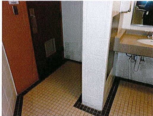
Photo 10: Maneuvering clearance is not currently provided at the entry to the upper level toilet rooms.
