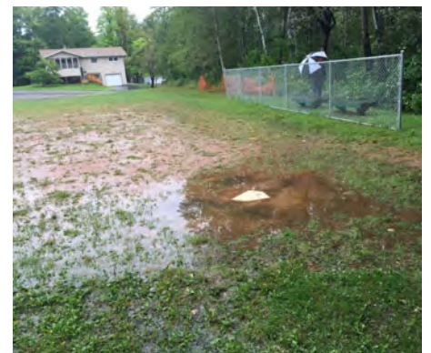
The existing ballfield has poor drainage
