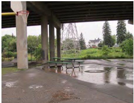
The existing surface of the basketball court is in poor condition
