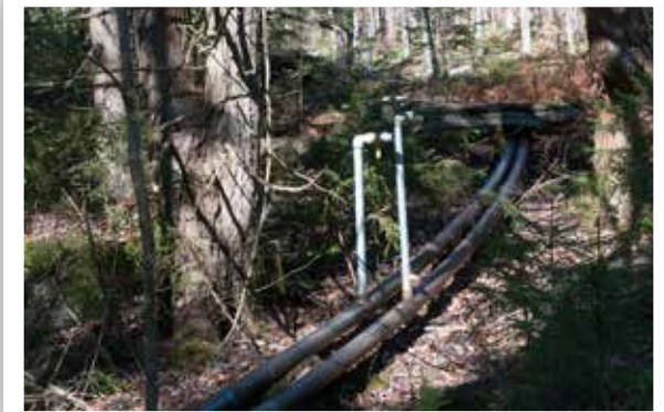
Snowmaking pipes running through the woods at Middlebury's Rickert Nordic Center. One pipe carries water and the other compressed air. Hoses connect hydrants to snow guns for making snow in place on the ski trail. The snowmaking system is used to cover 5km of their 50 km trail system with snow.
