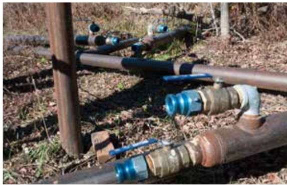
Top picture shows the holding pond, pump house and one of the snow guns at Middlebury's Rickert Nordic Center. The bottom picture shows system section intersections with connection valves. Short hoses are used to connect sections. One advantage of the air/water method is using the air to blow out water lines.
