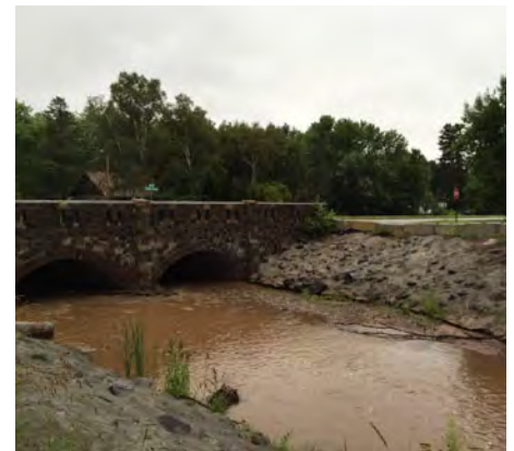
The historic bridge over Mission Creek will be replaced with the Hwy 23 reconstruction in 2016
