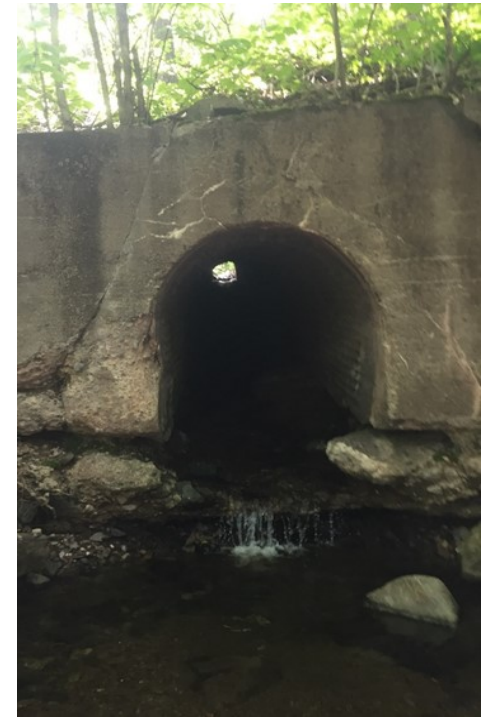
>>Photo Credit: Degraded box culvert, Jim Shoberg
