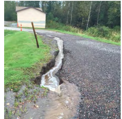
Erosion in the park is a major concern and poses a threat to public safety and water quality
