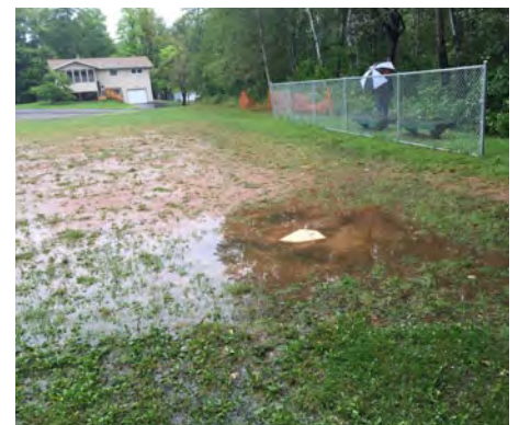
The existing ballfield has poor drainage
