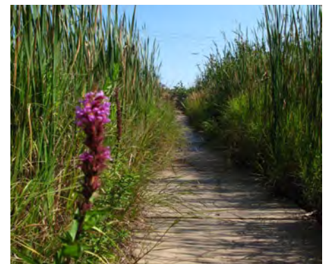
The floating boardwalk is becoming unstable, sinking with applied weight
