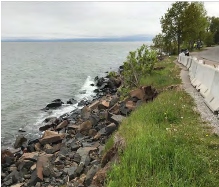
Figure 3: Photo documenting roadway and lakeshore damage. FEMA photo, October 2018.
