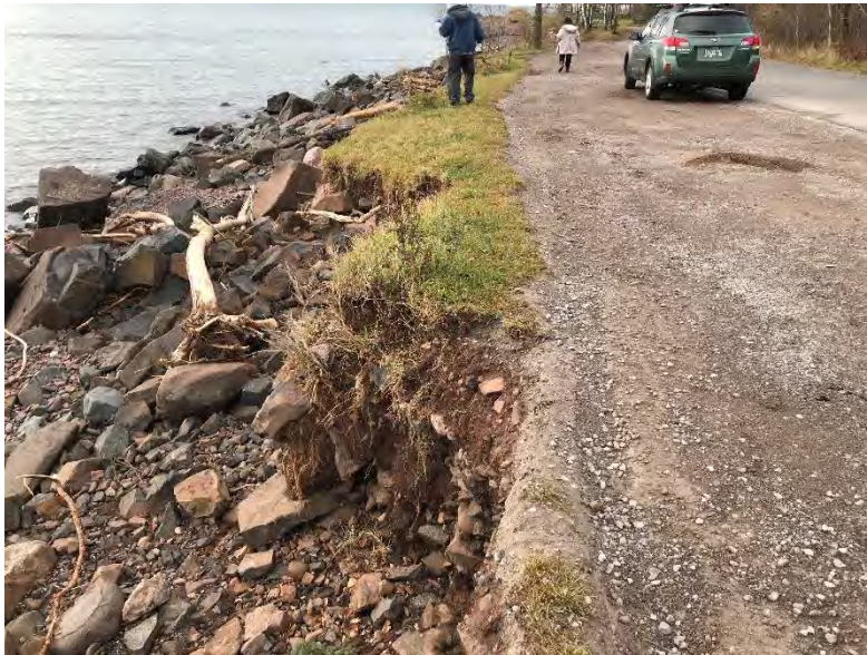
Figure 4: Photo documenting roadway and lakeshore damage. FEMA photo, October 2018.
